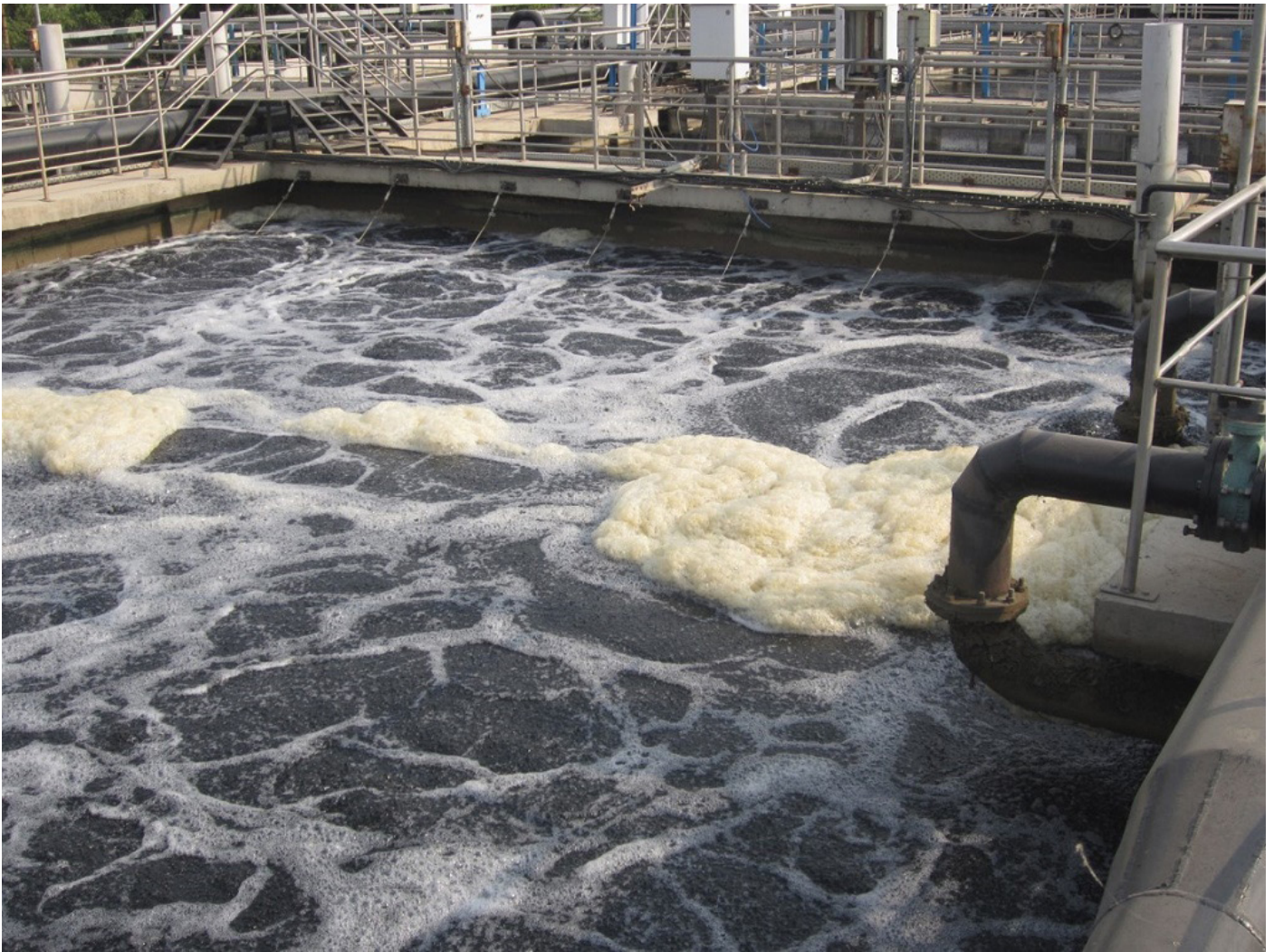
A wastewater treatment plant in Agra.
