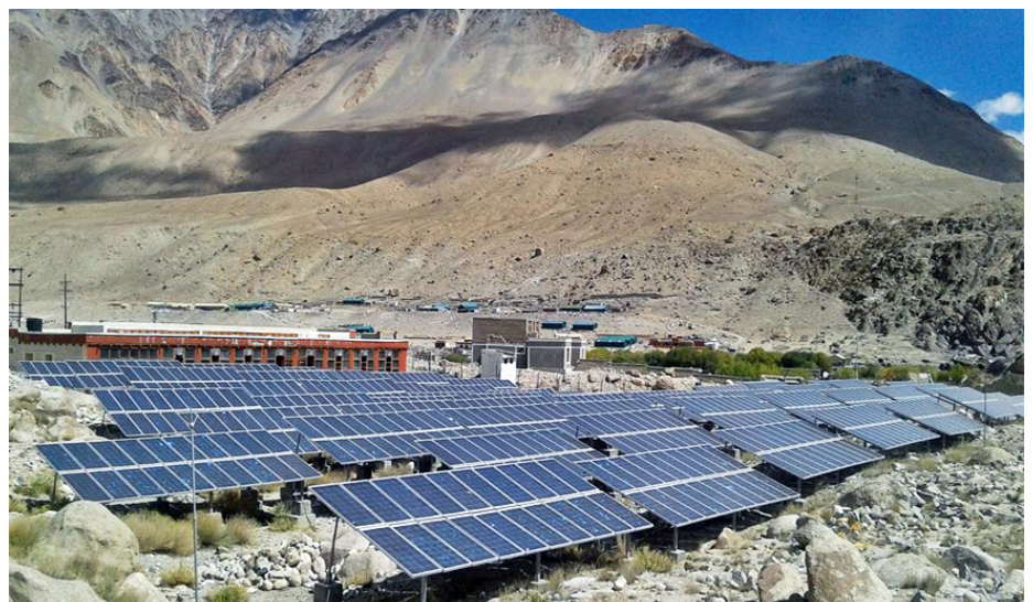
SPV off Grid Panels at Tangtse
